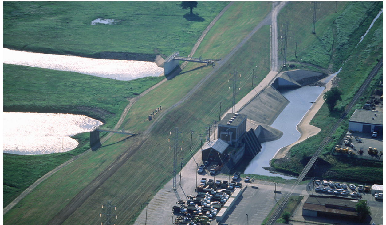
The Baker Pump Station on the east Levee.
